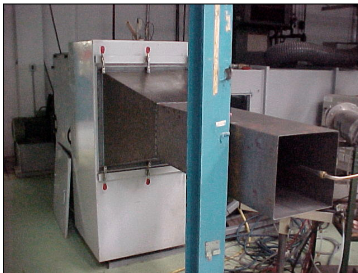
Figure 2 : View of the test facility before the installation of the tested ducts
